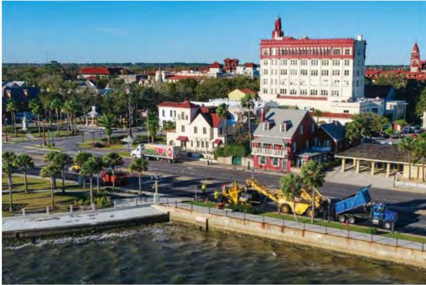
An average of 500,000 visitors to St. Johns County each month now get to enjoy the smooth and rut-resistant efforts of Duval Asphalt's project on State Route 5A along the bayfront in St. Augustine.
